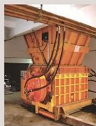
危险废物破碎 Hazardous pretreatment
